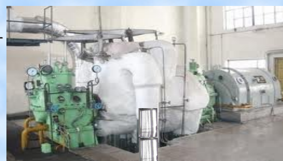
Direct Condensing Low Pressure Turbine Generator
